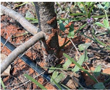
? Microcerotermes sp. damage, Termite (Termitoidea)
